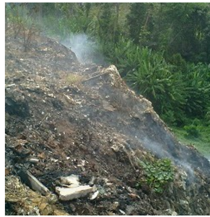
Plate A9-2 Slope Erosion
